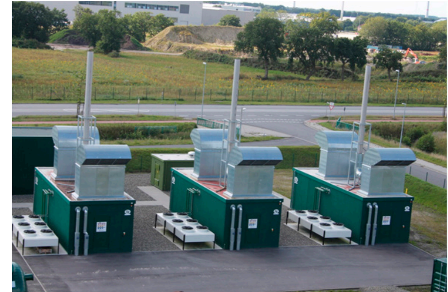
Figure A.55: CHP Generator
